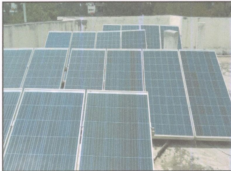
Photograph of Roof Top Solar PV Plant:
