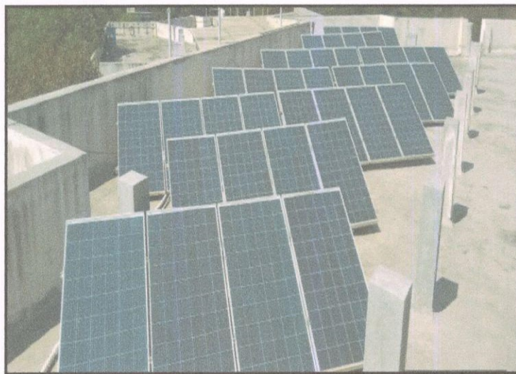
Photograph of Roof Top Solar PV Plant:
