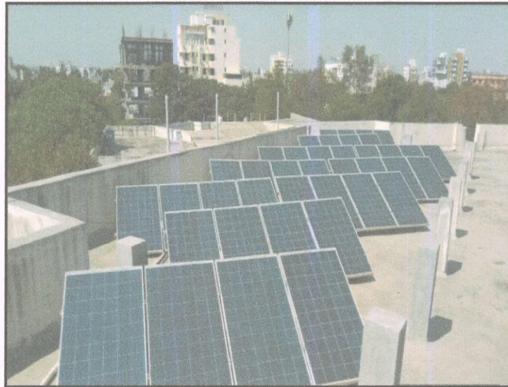
Photograph of Roof Top Solar PV Plant:
