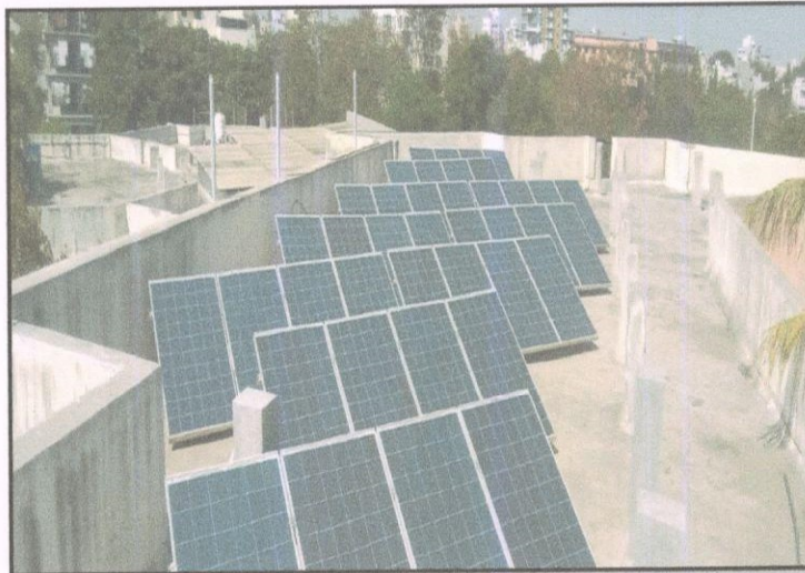
Photograph of Roof Top Solar PV Plant:
