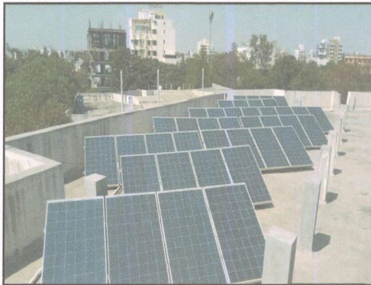
Photograph of Roof Top Solar PV Plant:
