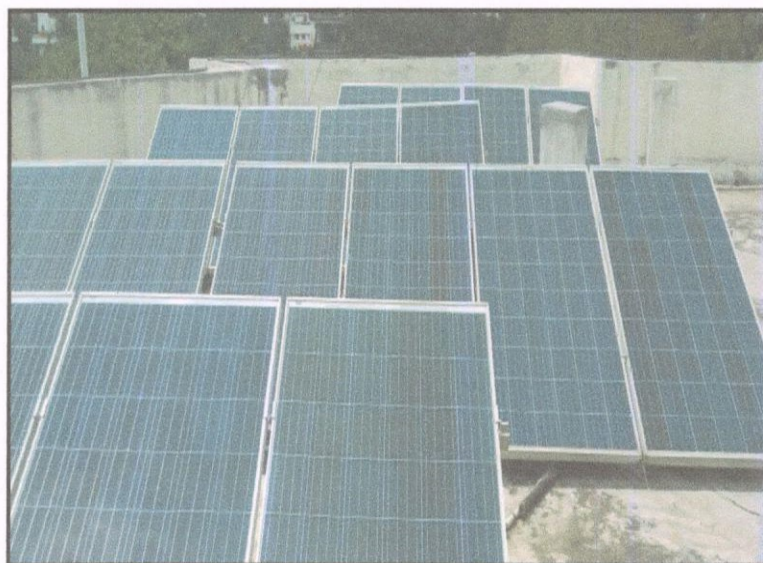
Photograph of Roof Top Solar PV Plant:
