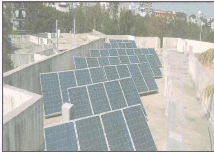
Photograph of Roof Top Solar PV Plant:
