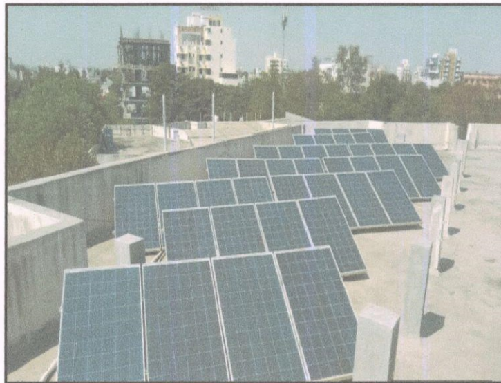
Photograph of Roof Top Solar PV Plant:
