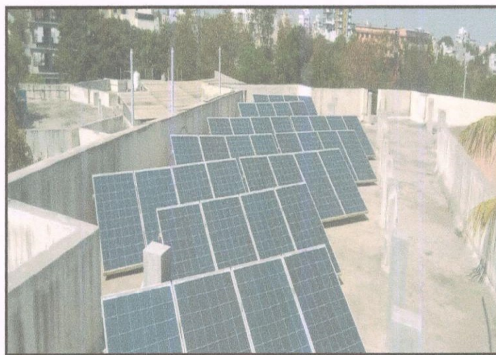
Photograph of Roof Top Solar PV Plant:
